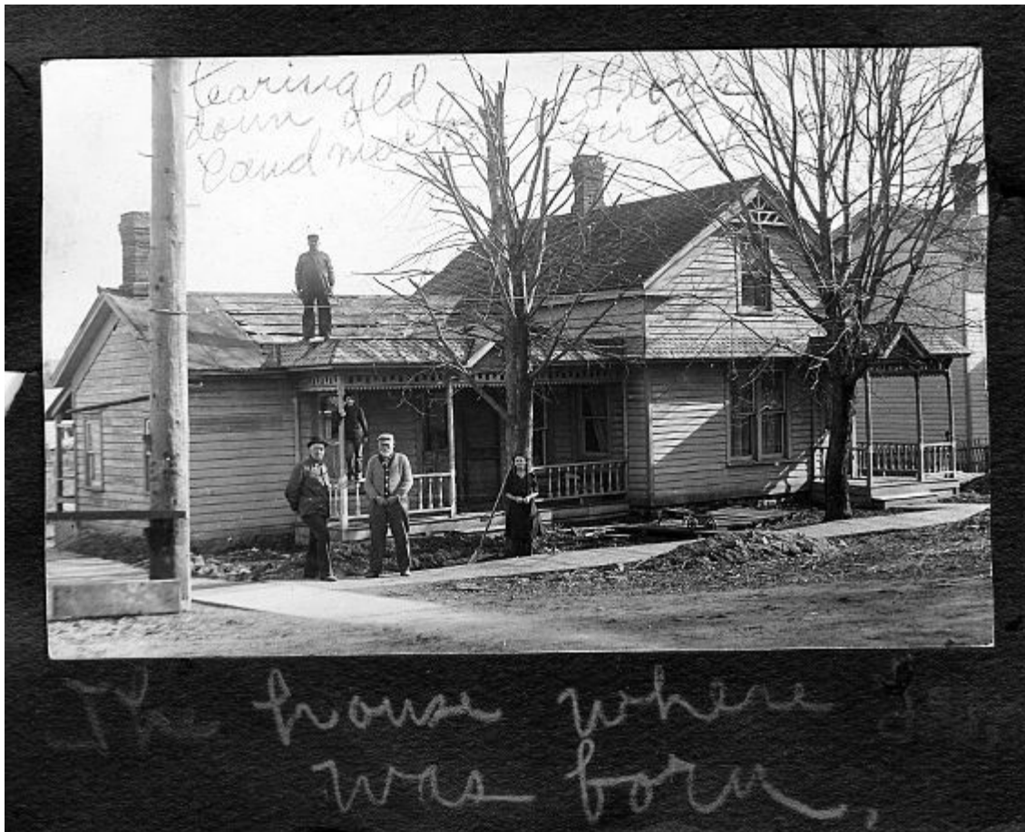
Undated photo of the first Breylinger home in Monticello when it was being torn down. Leon was born there.
