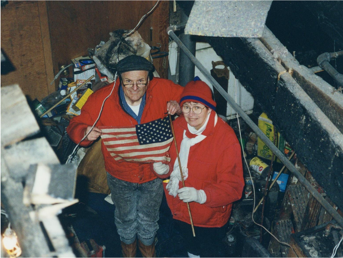
Mickey and Fred after the house fire in 1996; photographer looking down from the living room into the basement at Fred and Mickey after a gas explosion that left a 10-foot hole in the living room floor.
